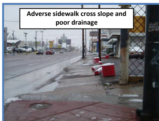
Figure 13: Examples of Poor Sidewalk Condition along West Colfax
